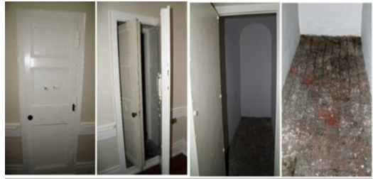
Views of original 1833 Vault. Approximate dimensions: 5 feet wide, 8 feet tall (at ceiling peak), 12 feet deep.
